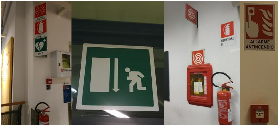
Figure 2 - The use of fire safety signs in Italian buildings
